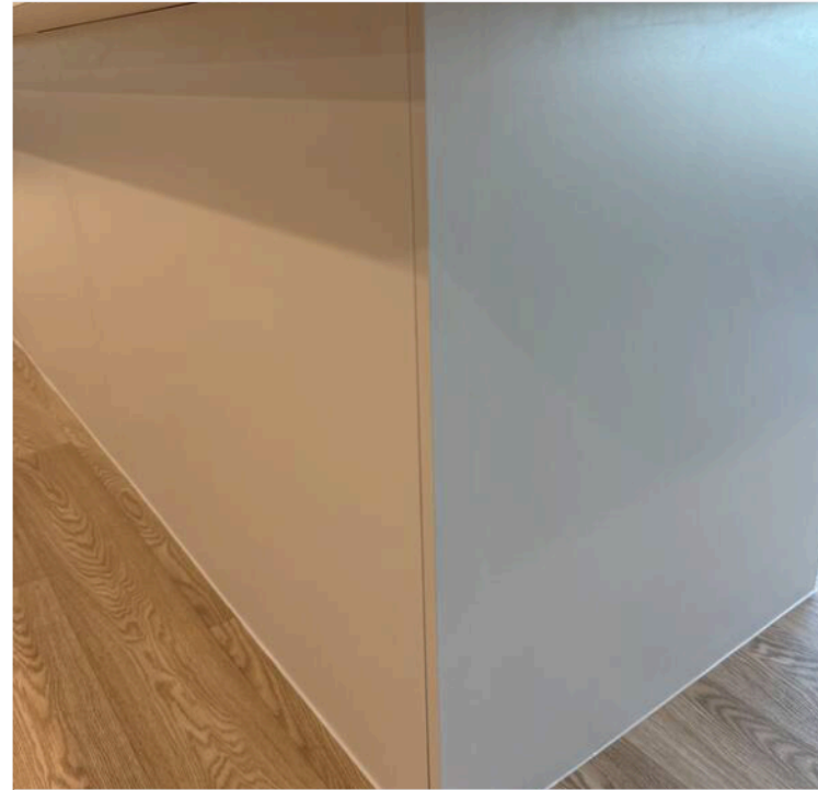
Ref 20a · #20 Back panel/end panel not fitted correctly for: Joiner
