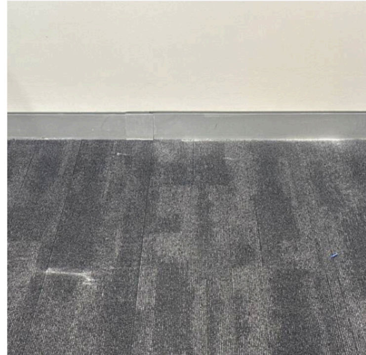
Ref 11a · #11 Skirting patch imperfect for: Builder
