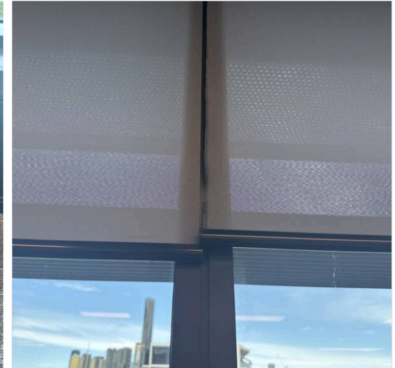
Ref 4a · #4 Blinds frayed and not in alignment for: Blinds installer
