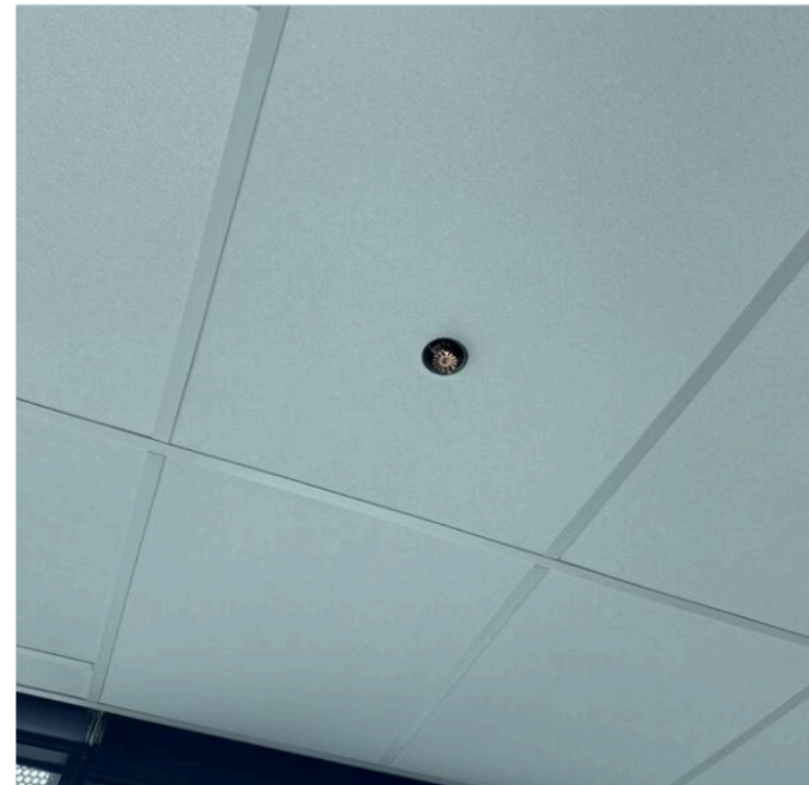
Ref 15a · #15 Suite 2 - Missina fire sprinkler cover for: Builder
