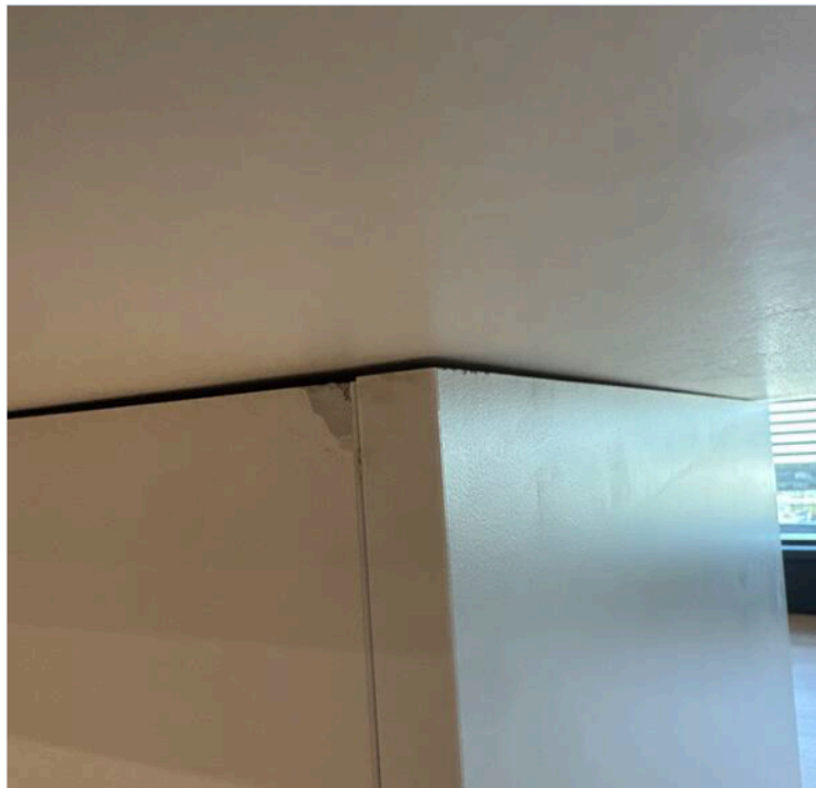
Ref 20c · #20 Back panel/end panel not fitted correctly for: Joiner
