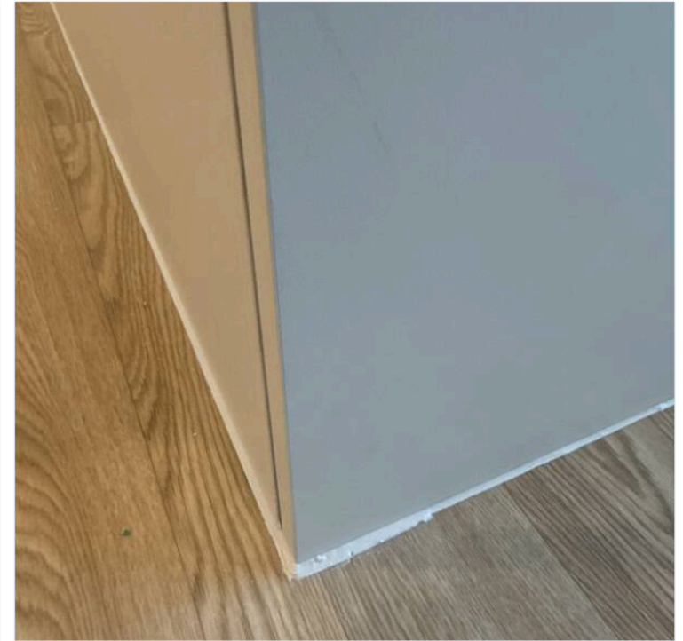
Ref 20b · #20 Back panel/end panel not fitted correctly for: Joiner
