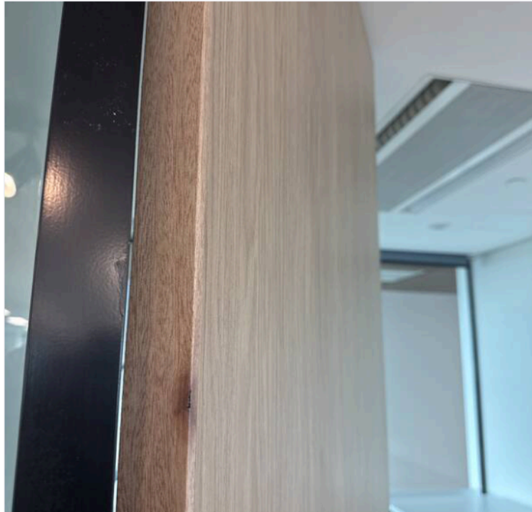
Ref 9a · #9 Imperfection in door for: Cleaners
