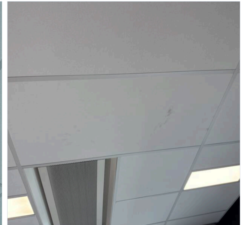
Ref 16a · #16 Replace/clean ceiling tile for: Carpenters
