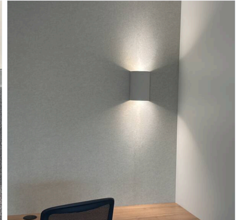
Ref 12a · #12 Quiet room 1,2&3 acoustic panel joint under light for: Builder
